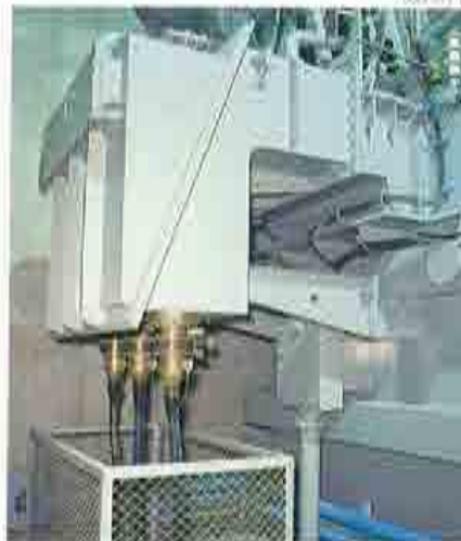
Photo 4 Oil-filled type cable junction box
