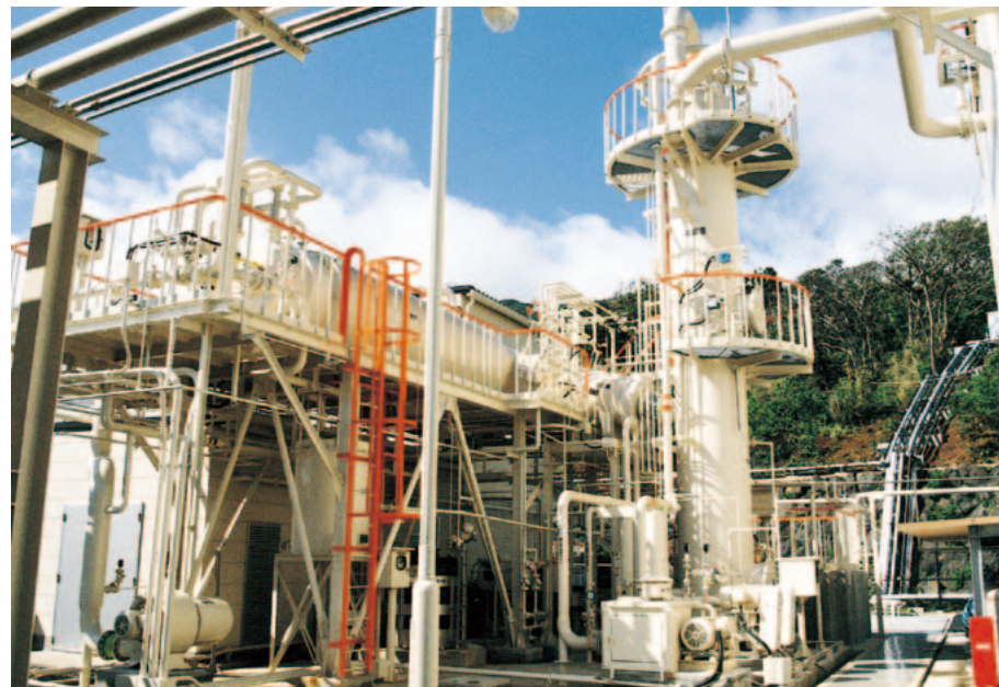
H 2 S abatement system
