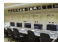
Plant monitoring and control system
