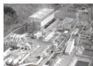
2017 Delivered one of Japan's largest geothermal binary equipment (5,050 kW for the Takigami Binary Geothermal Power Plant)
