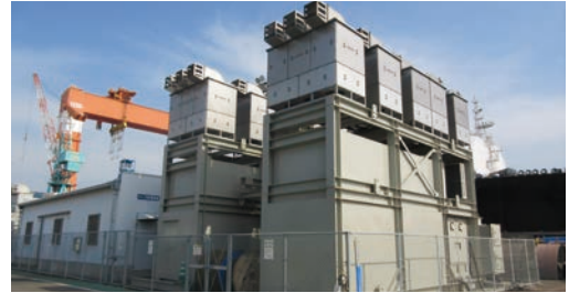
Onshore power supply system (exterior view)
