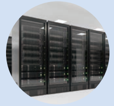
Power supply and facility systems
