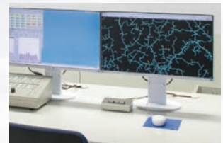
Energy management systems (EMS)
