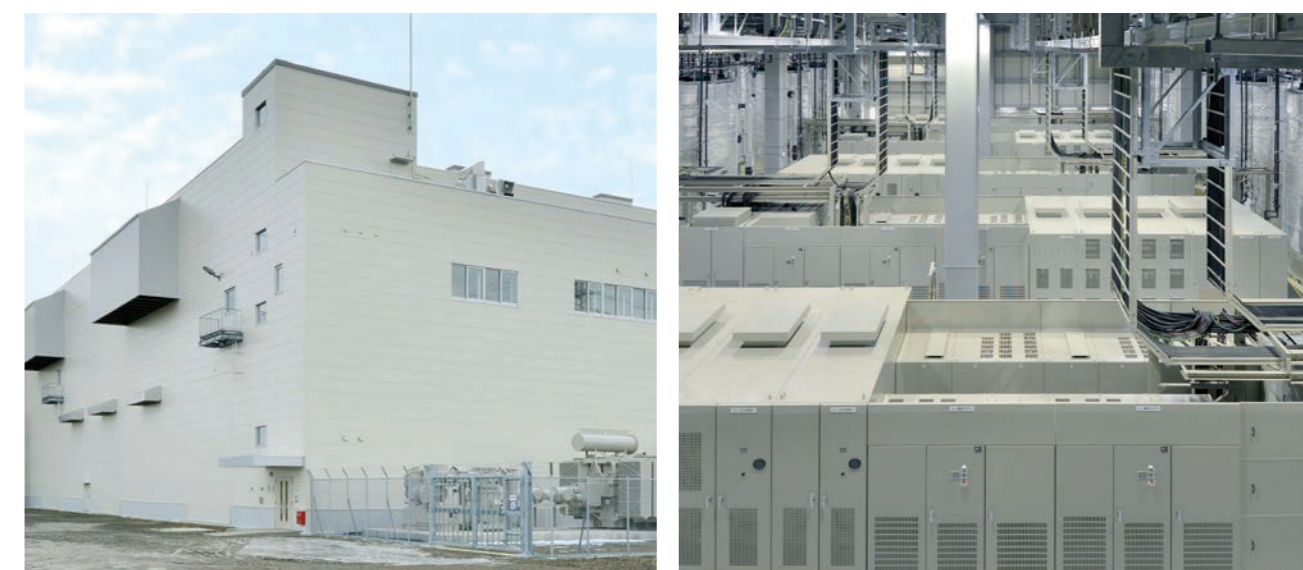
Minami-Hayakita Substation (Left: exterior view of the building Right: Fuji Electric power conditioning system inside the building)
