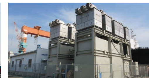
Onshore power supply system (exterior view)
