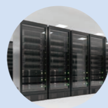
Power supply and facility systems
