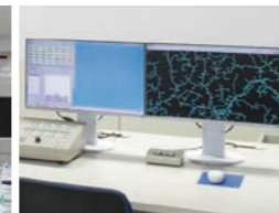
Energy management systems (EMS)
