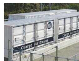
Power storage systems
