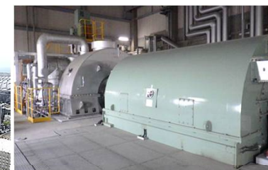
Steam turbine and generator
