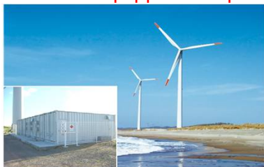
Nishime wind power plant (288 kWh lead-acid storage battery, 22 kWh LiB)
