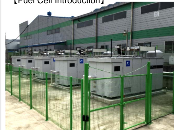
Five 100 kW fuel cells introduced Yuil Industry facility in South Korea (completed in 2017)
