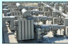
Industrial substations (Power receiving and distribution substation equipment)
