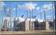
Power grid substations (Large-capacity transformers)
