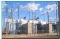
Power grid substations (Large-capacity transformers)
