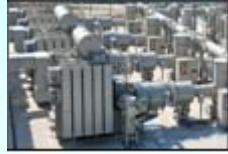
Industrial substations (Power receiving and distribution substation equipment)
