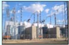
Power grid substations (Large-capacity transformers)
