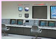
Instrumentation systems (Control systems)
