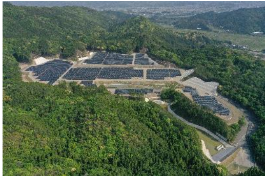
Solar power generation system for Nobeoka Kujiraike (under construction) (Photograph provided by Nobeoka Solar power)
