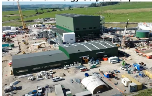
Tauhara Geothermal Power Plant (under construction) (Photograph provided by Contact Energy Ltd.)
