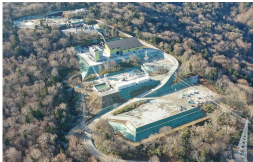
Appi Geothermal Power Station (under construction) (Photograph provided by Appi Geothermal Energy Corporation)
