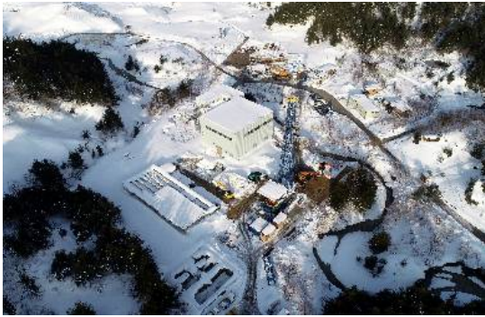
Onikobe Geothermal Power Station (under construction) (Photograph provided by Electric Power Development Co., Ltd.)
