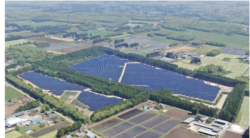
Aoki Solar Power Plant (under construction) (Photograph provided by First Solar Japan Co., Ltd.)
