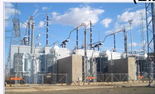
(High-capacity transformers) Power grid substations
