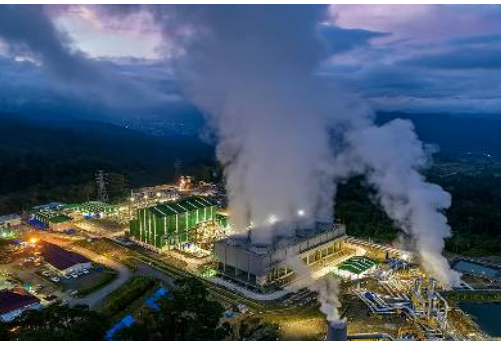
Muara Laboh Geothermal Power Plant (Photograph provided by PT. Supreme Energy Muara Laboh)
