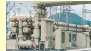
GISs (gas insulated switchgears)
