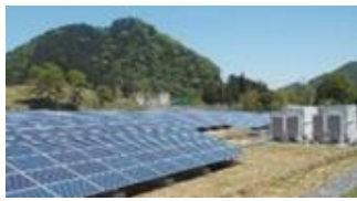
Solar power PCSs
