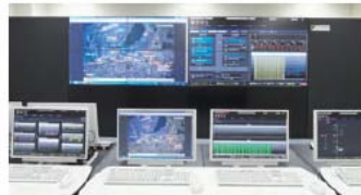
Cluster Energy Management System
