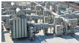
Power receiving and transforming facilities
