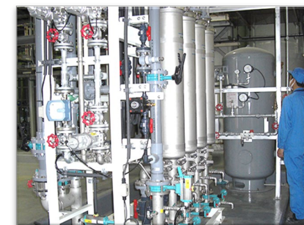
Grinding Debris Recovery Membrane Unit
