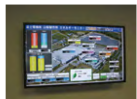
Energy monitor displays the energy being used
