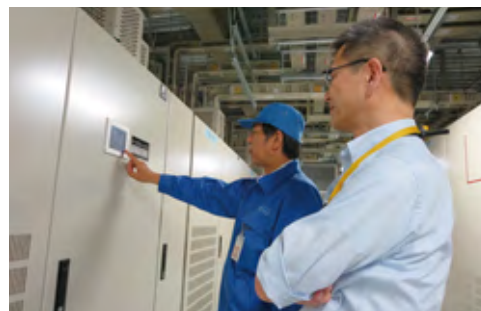
Inspecting a UPS unit
