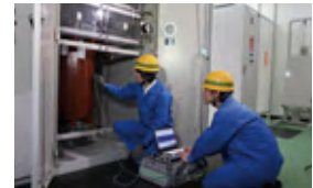
Service activities involve making proposals for overall plant optimization
