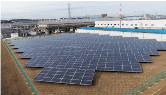
Solar power generation system introduced at a Smart Factory Initiative model factory (Mie Factory)
