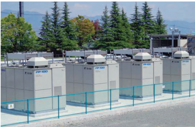
Fuel cells installed at the Yamanashi Branch Factory under the Smart Factory Initiative
