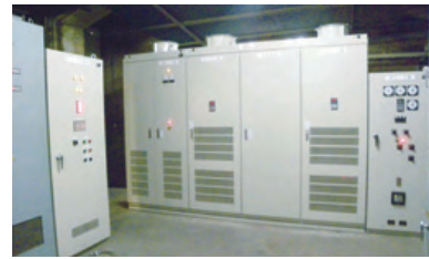
The drive control system (inverter) controls kiln rotation
