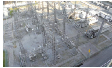
Power receiving and distribution substation equipment
