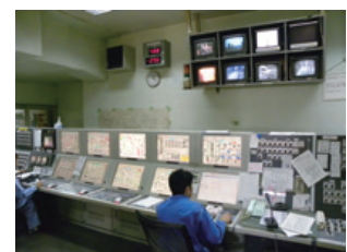
The production monitoring control system visualizes cement production processes
