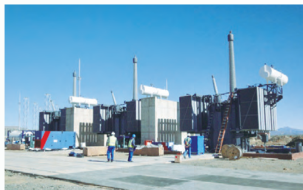
Transforming equipment being installed onsite for Kappa Substation of Eskom Holdings, a state owned-power producer in the Republic of South Africa
