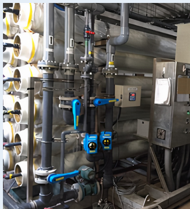
Wastewater recovery system
