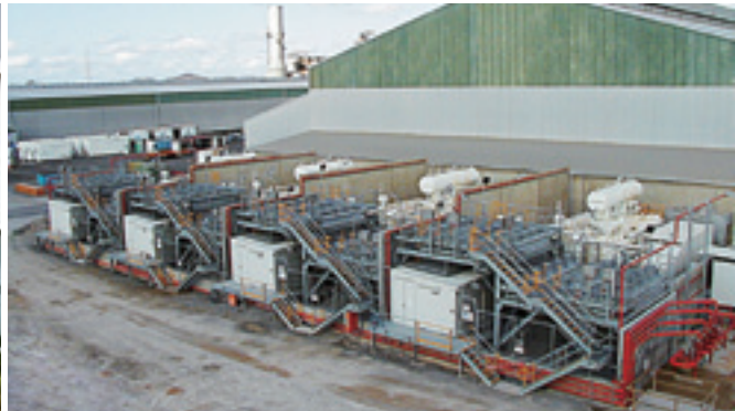
High-capacity rectification equipments
