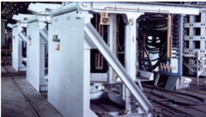
Induction heating equipments
