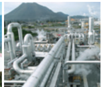
Kawerau Geothermal Power Plant (New Zealand)
