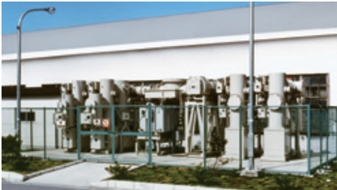
Electric substation equipments
