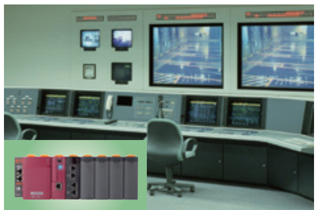
Plant monitoring control system
