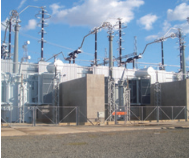
Substation equipments (transformers)
