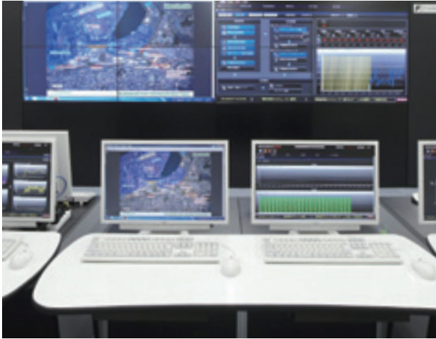
Cluster Energy Management System(CEMS)
