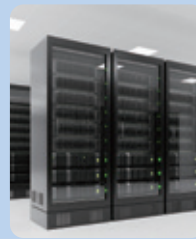
Power supply and facility systems
