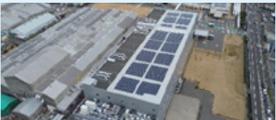
Solar power generation equipment at Suzuka Factory
