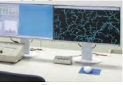
Energy management systems (EMS)
