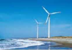
Wind power generation
