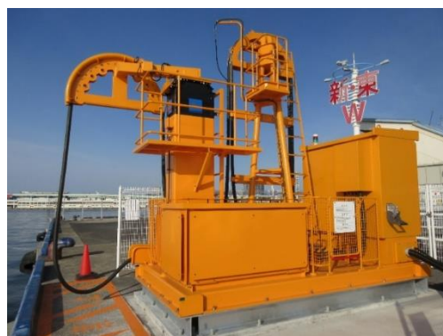
Capable management system delivered to Kobe City (operation commenced in April 2024)
