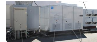
120kW demonstration equipment
