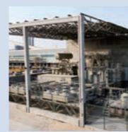
High-capacity rectification equipment
