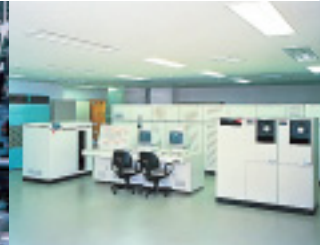
Power Industry Radiation Monitoring Systems
