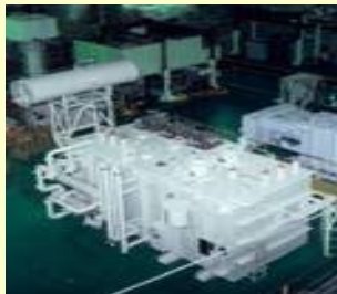
Electric furnace power supplies
