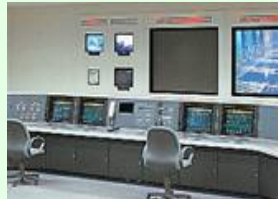
Plant control systems
