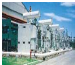
High-capacity rectification equipment (No.2 global share)
