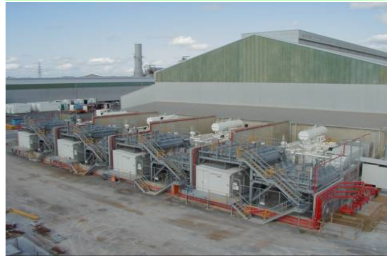
Australia— High-capacity rectification equipment for aluminum smelter
