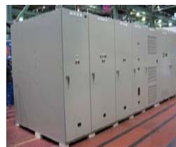
High-voltage drop/dip compensators
