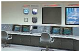
Plant control systems
