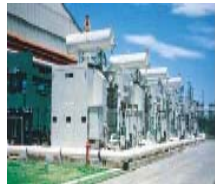
High-capacity rectification equipment
