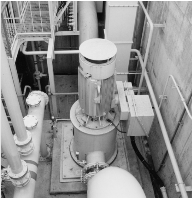
Fig.10 Exterior view of the hot well pump
