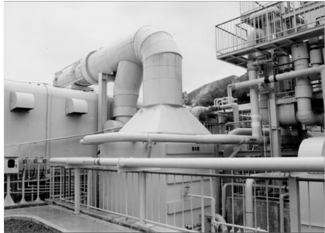
Fig.8 Exterior view of the condenser
