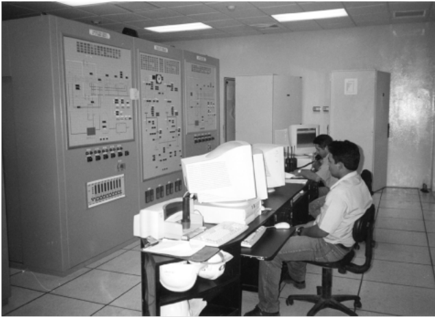
Fig.10 Plant control room
