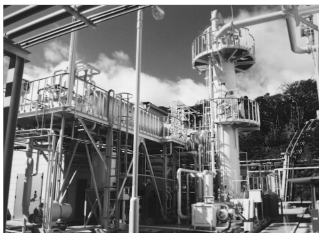
Fig.9 Exterior view of the H 2 S abatement system
