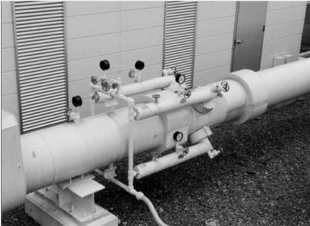
Fig.5 Exterior view of the venturi tube
