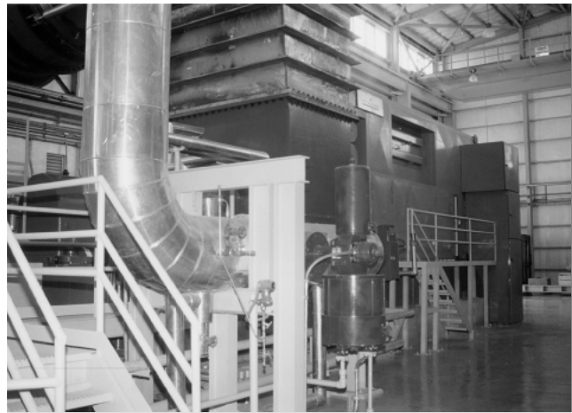
Fig.5 Turbine and generator
