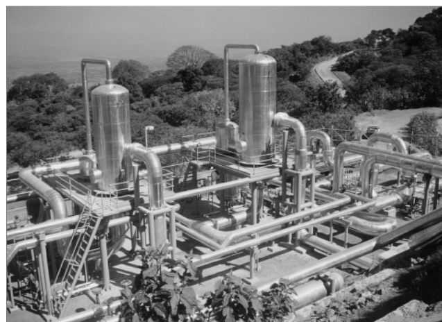
Fig.4 TR-5 wellpad separators
