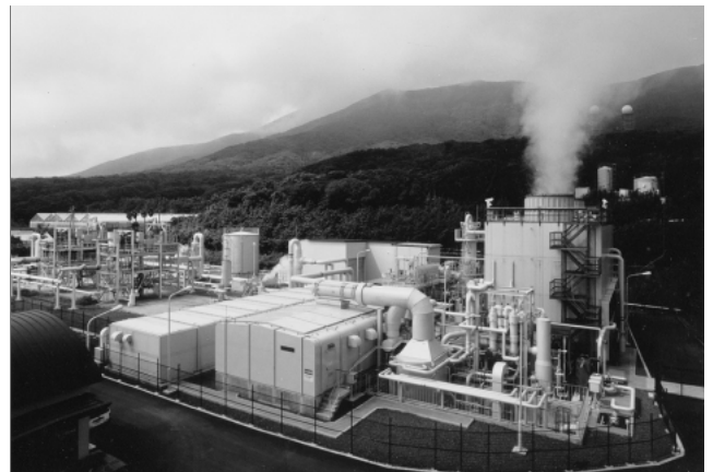
Fig.1 Overview of Hachijo-jima Geothermal Power Plant
