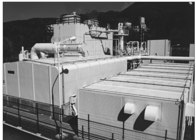
Fig.14 View of the package-type electrical control room
