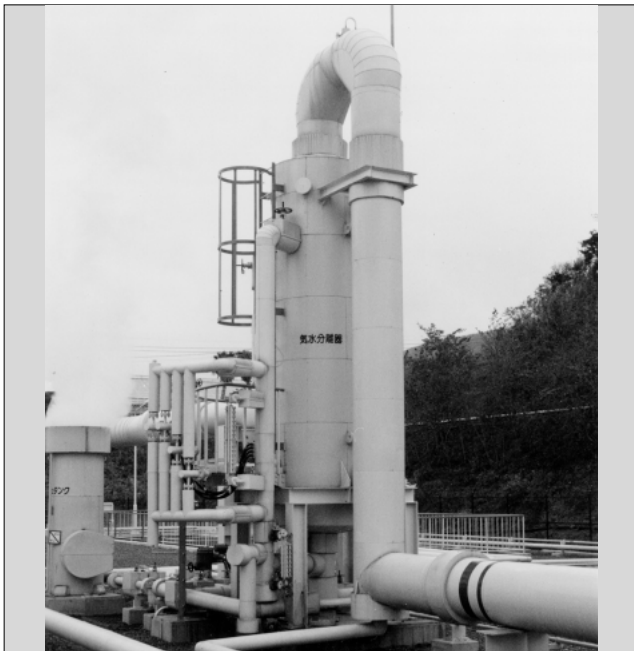
Fig.4 Exterior view of the separator
