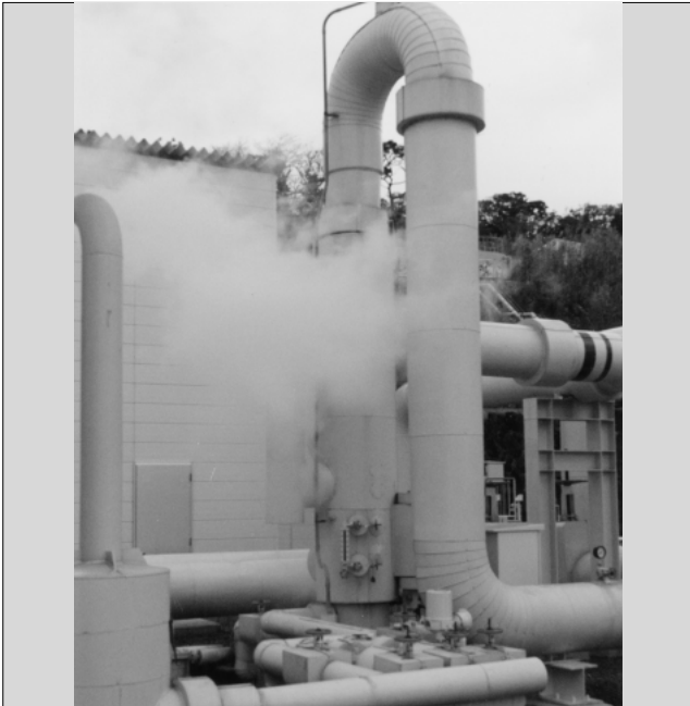
Fig.6 Exterior view of the mist separator
