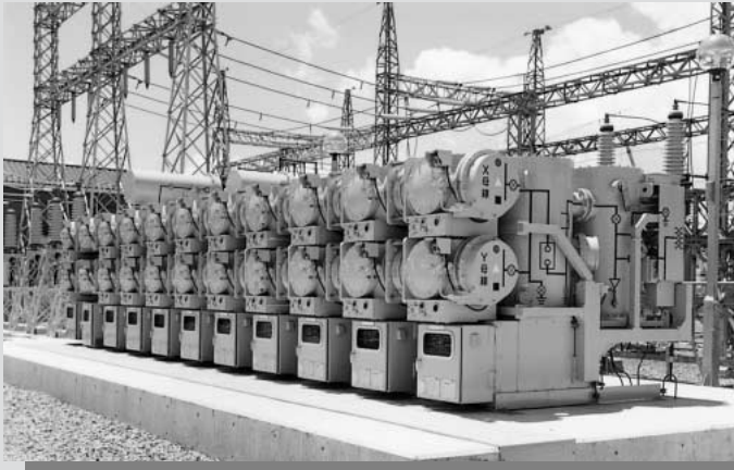
72.5kV three-phase-encapsulated GIS
