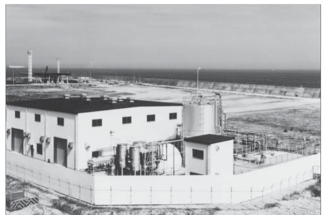
Fig.2 Exterior view of power generating facility using biogas from garbage
