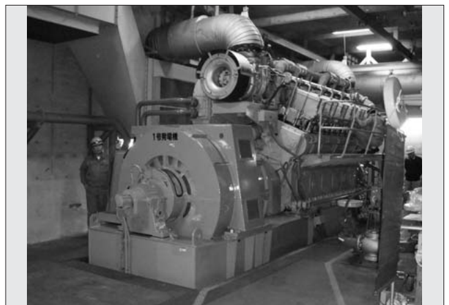
Fig.42 Emergency power generator of Joyo
