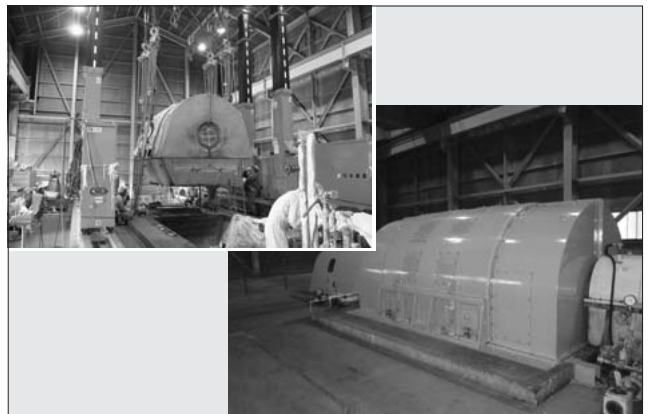
Fig.41 Transferring out of the former power generator stator and installation of the new power generator stator
