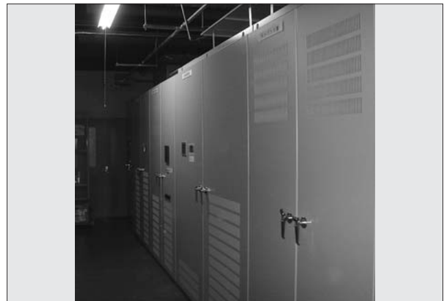
Fig.35 Medium-voltage UPS unit using lithium-ion capacitor
