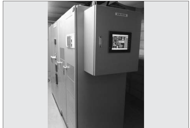
Fig.28 AC/DC converter and monitoring control system
