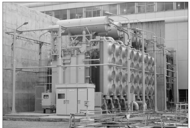
Fig.24 1,050 MVA main transformer
