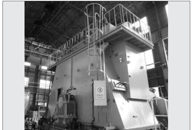
Fig.40 7,700 kW, 34P synchronous motor under factory test
