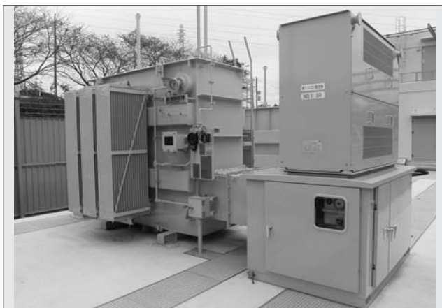
Fig.27 66 kV power-receiving and direct-current transforming facility
