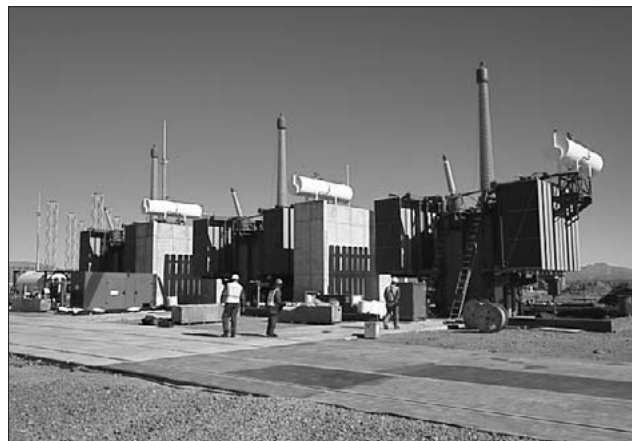
Fig.25 765 kV, 400 Mvar shunt reactor
