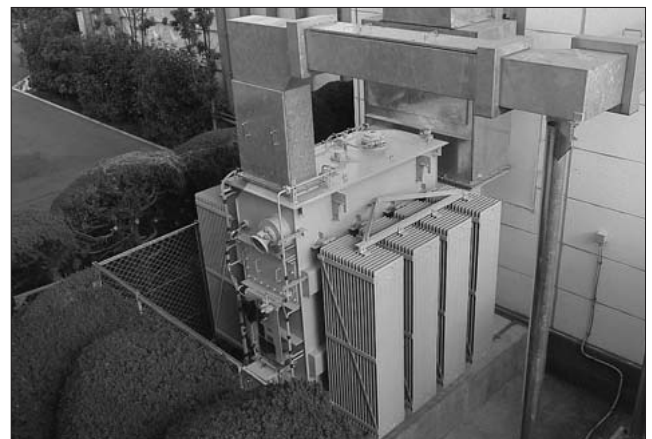
Fig.36 Ecore Trans (22 kV to 6,000 kVA)
