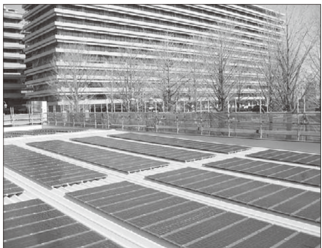
Fig.5 Solar cell on roof of bicycle parking lot, Kumamoto prefectural government
